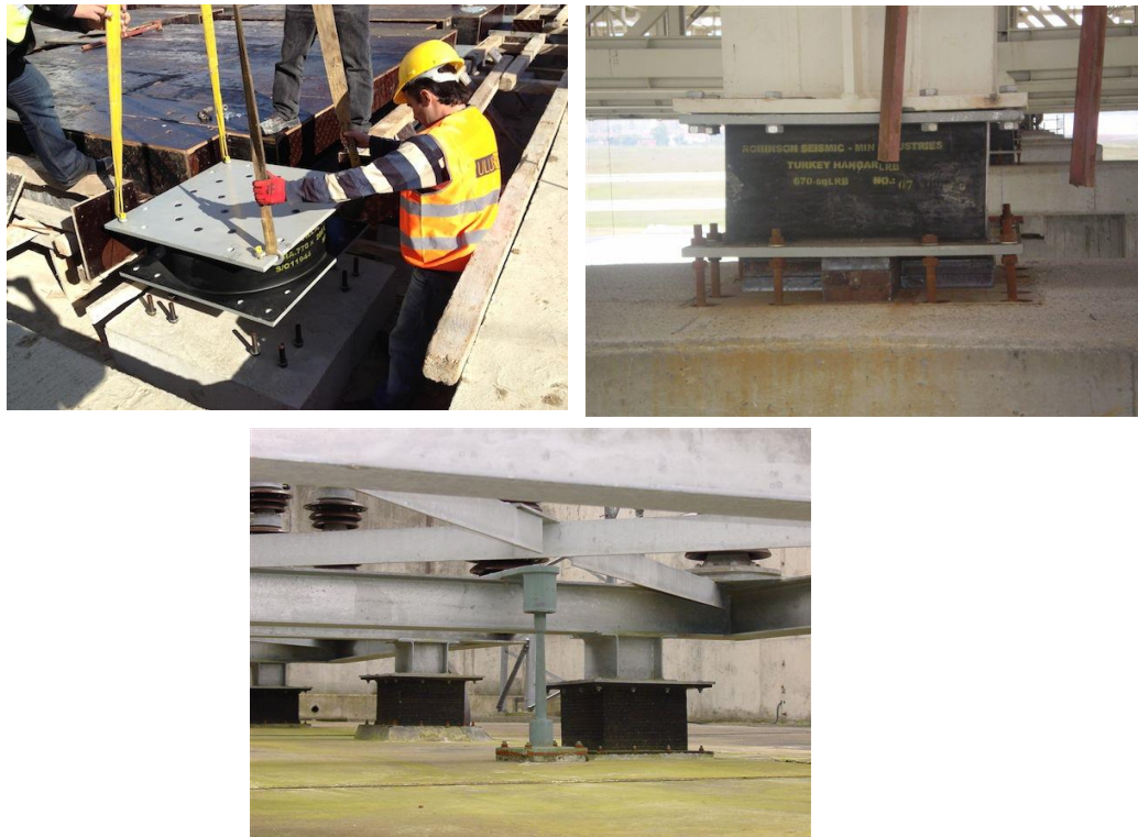
Figure 2-5. The application of base isolation, Sabiha Gokcen Airport in Turkey,
